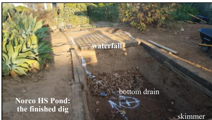
Norco HS Pond: the finished dig Bordered by railroad ties, the digging is done. Marking is for a bottom drain; there will be a skimmer at the near end, a waterfall at the far end. A liner has been donated. Kids still need to pour a 3' walk on one side and make space for the equipment.
